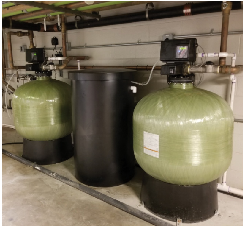
A water softening system works to remove minerals, iron and other deposits from the water. This filters the water to prevent impurities from clogging the hundreds of misting jets in the green line trench.
