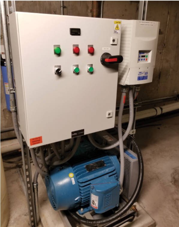
A control box contains the computer system that ensures the pump carrying water to the mist jets has the correct pressure for producing the special effects.
